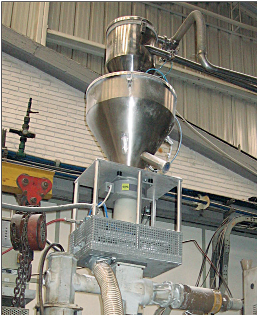
Metal separator installed at the material infeed.
